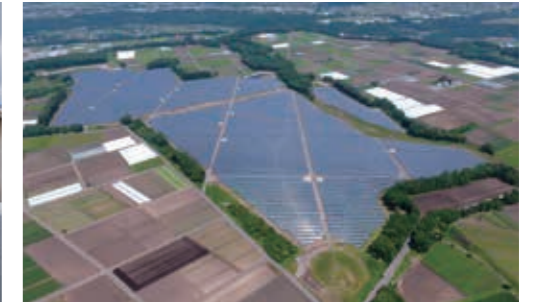
Solar power equipment in Hitachi Showa Village
