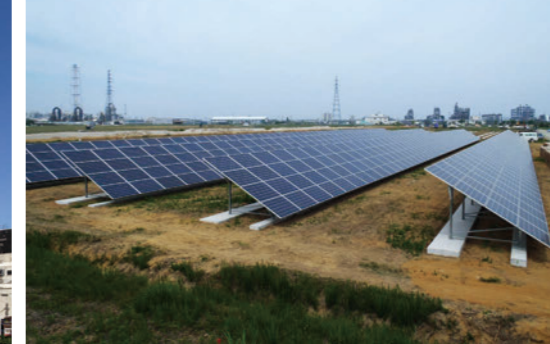
Soma Solar Power Plant (Fukushima, 2013)
