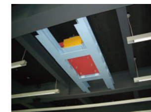
Tuned mass damper
