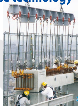
Construction using the precast concrete method (an example of the FHRC construction method)
