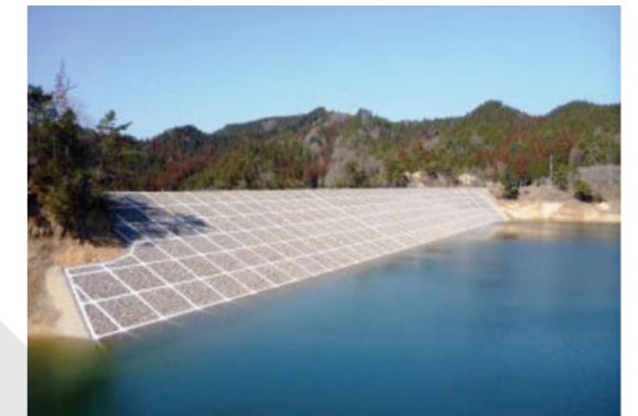
Example of fill dam embankment repair using the stabilized muddy soil embankment method
